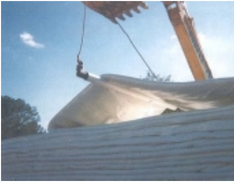
A trackhoe was used to lift the heavy liner to relieve stress during the inversion process.
